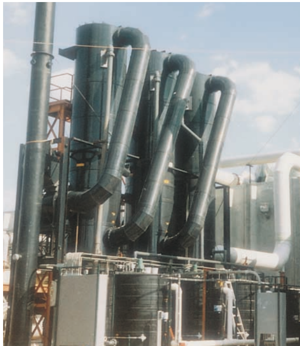
Tri-NO x ® Multi-Chem ® plant constructed of black, UV-stabilized polypropylene with external recirculation systems and catwalk access assembly.
