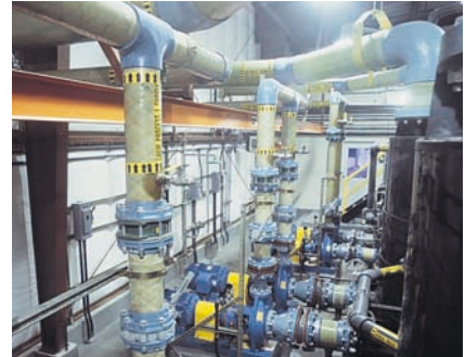
Multi-stage scrubber pump room.
