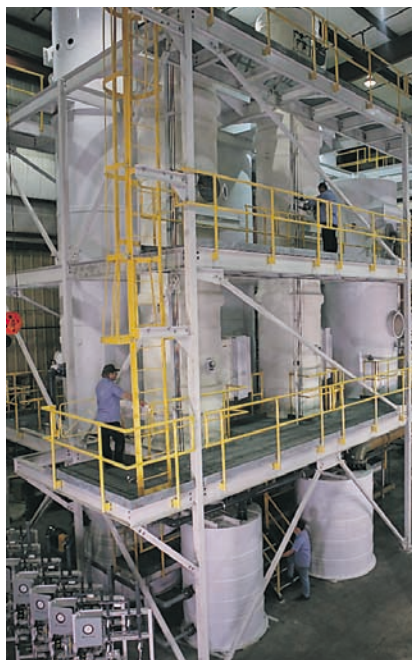
Multi-stage scrubber system (Tri-NO x ®) constructed of polypropylene and fiberglass, with catwalk access.
