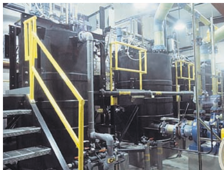
External recirculation tank farm.
