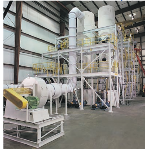
Fiberglass-constructed, two-stage HCl scrubber with dual fans and catwalk assembly.
