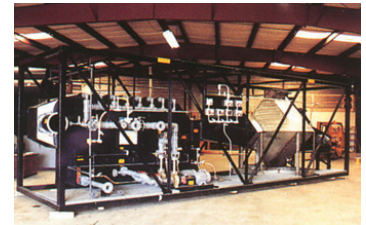
Horizontal multi-stage wet chemical odor control with carbon bed.
