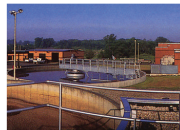
Wastewater treatment plant
