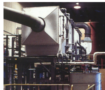
Multi-stage horizontal NO x scrubber applied to steel pickling line.
