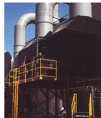
A 60,000 CFM AnoVent system venting a bright dip operation.
