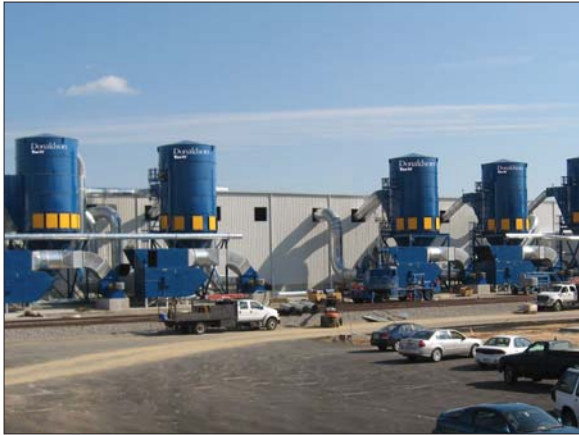
776RF at wood furniture plant
