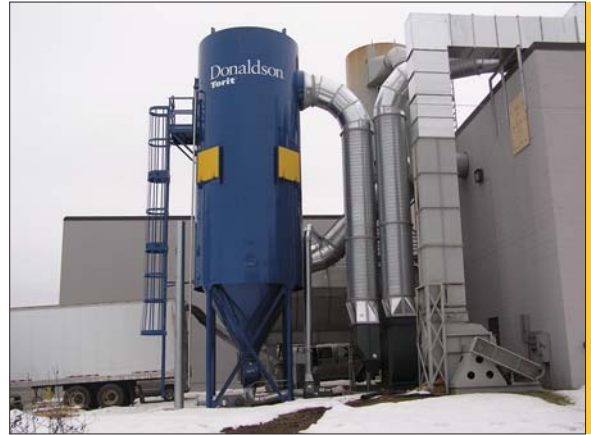
376RF at cabinet shop
